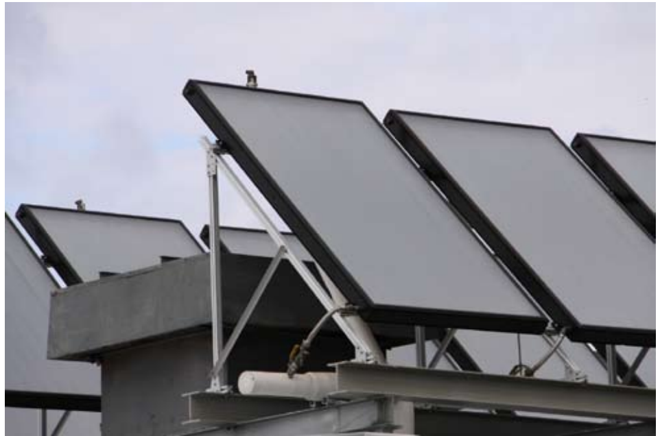
Figure 2 Flat panel array
