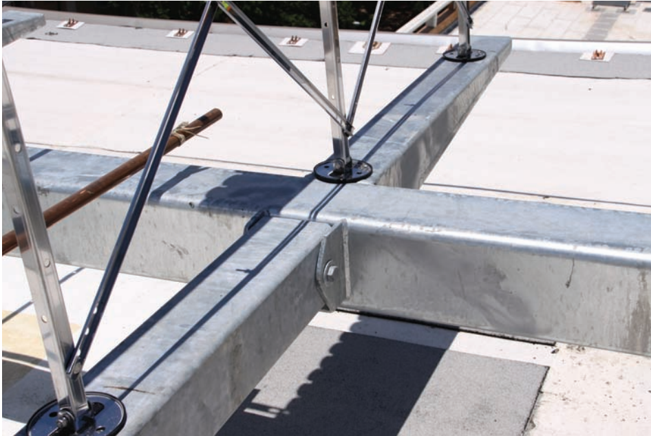
Figure 1 Example of structural steel supports Source: Cinco Solar
