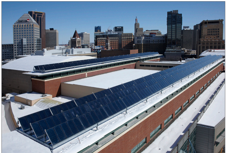
Solar water heating panels installed at the St. Paul River Centre, MN
